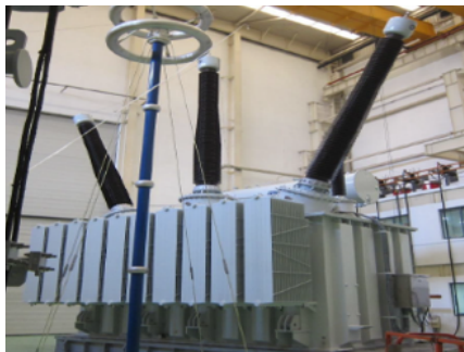
Serbia | 400kV variable shunt Reacto
