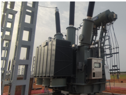
Senegal | 225kV variable shunt Reactor
